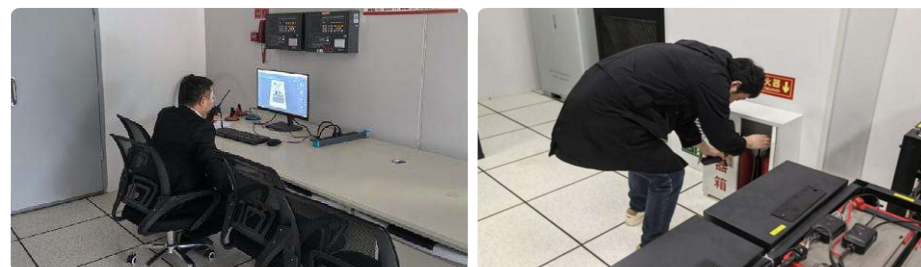
Server Room Fire Emergency Drill
